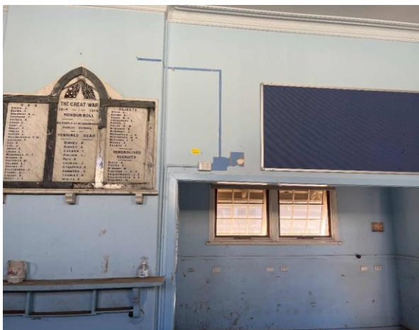
Line ID 58: Internal, Building F, Throughout, Walls, Light Blue Paint - Lead Detected (0.082% w/w)
