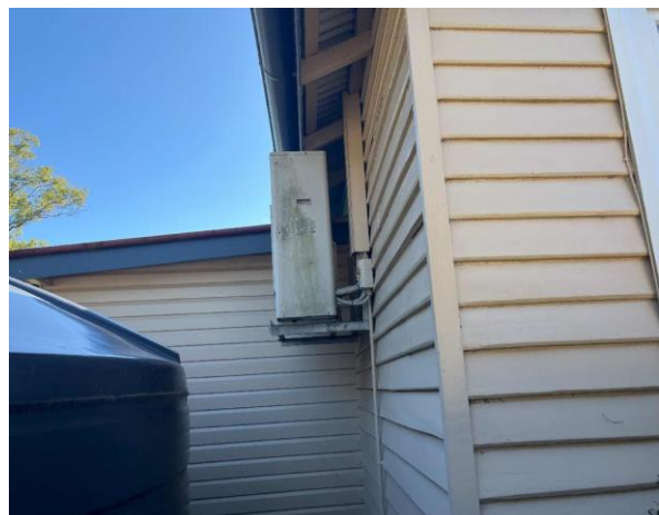
Line ID 71: External, Building E, Western Side, Daikin Air Conditioning unit, R410A Hydrofluorocarbon (HFC) - Non ODS Refrigerant
