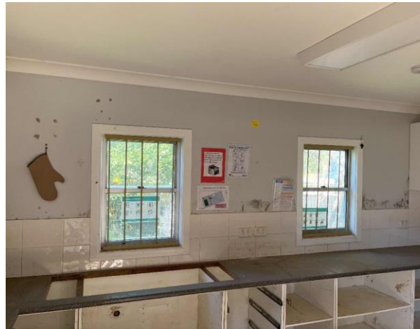
Line ID 48: Internal, Building C, Throughout, Walls, Blue Paint - Lead Detected (<0.005% w/w)
