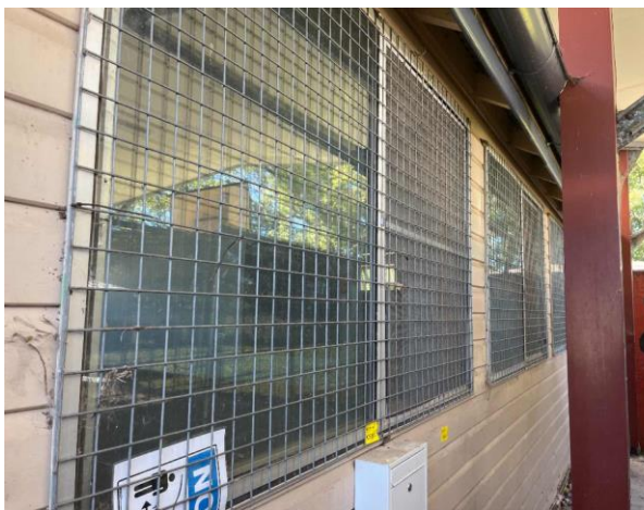
Line ID 5: External, Building E, Northern Side, Aluminium Framed Windows, Mastic - Chrysotile Asbestos Detected
