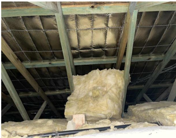
Line ID 68: Internal, Building J, Throughout, Ceiling Void, Sarking - Suspected SMF
