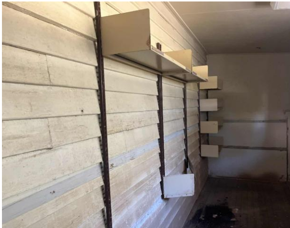
Line ID 54: Internal, Building E, Western Room, Eastern Wall, Beige Paint - Lead Detected (0.04% w/w)
