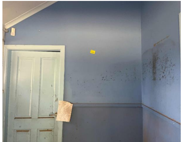
Line ID 55: Internal, Building F, North West Room, Walls, Blue (Dark) Paint - Lead Detected (<0.005% w/w)
