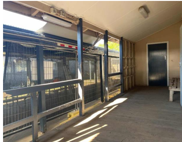
Line ID 36: External, Building E, Throughout, Posts, Railings and Doors, Blue (Dark) Paint - Lead Detected (0.009% w/w)
