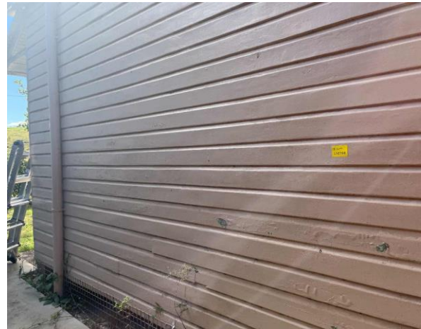
Line ID 32: External, Building A, Throughout, Walls, Beige Paint - Lead Detected (0.13% w/w)
