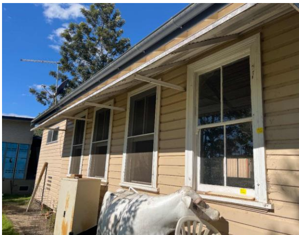
Line ID 33: External, Building A, Throughout, Window and Door Frames, White Paint - Lead Detected (2.8% w/w)
