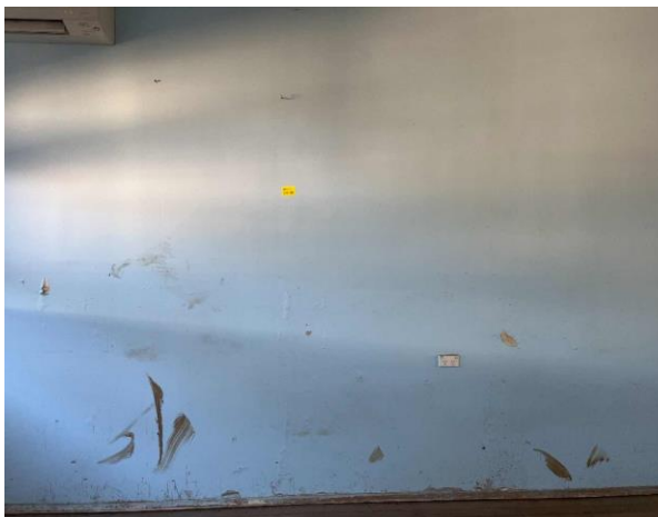
Line ID 52: Internal, Building E, Throughout, Walls, Blue (Light) Paint - Lead Detected (0.086% w/w)
