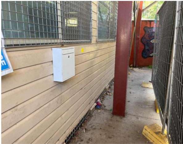
Line ID 37: External, Building E, Throughout, Walls, Beige Paint - Lead Detected (0.04% w/w)
