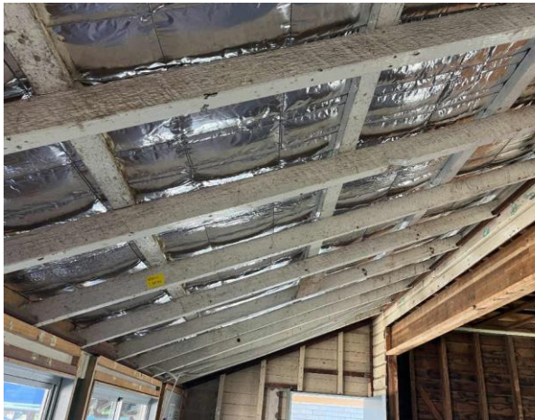
Line ID 47: Internal, Building A, Throughout, To Rafters, White Paint - Lead Detected (0.80% w/w)
