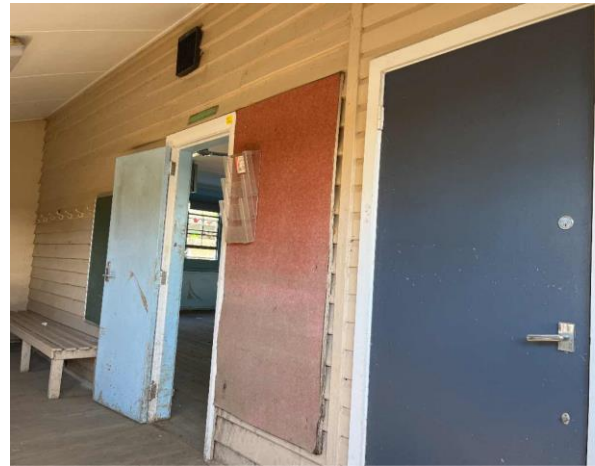
Line ID 38: External, Building E, Throughout, Windows and Door Frames, White Paint - Lead Detected (0.03% w/w)
