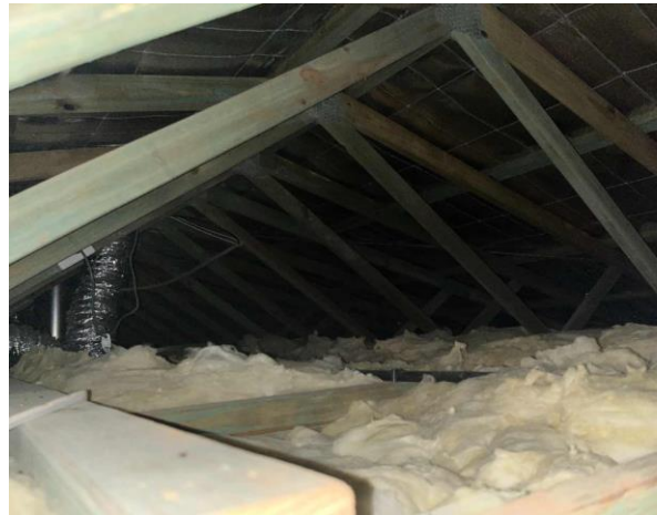
Line ID 67: Internal, Building J, Throughout, Ceiling Void, Insulation Batts - Suspected SMF
