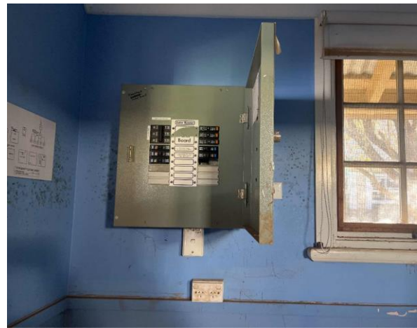
Line ID 25: Internal, Building F, North West Room, Switchboard, HRC Fuses - Suspected Asbestos
