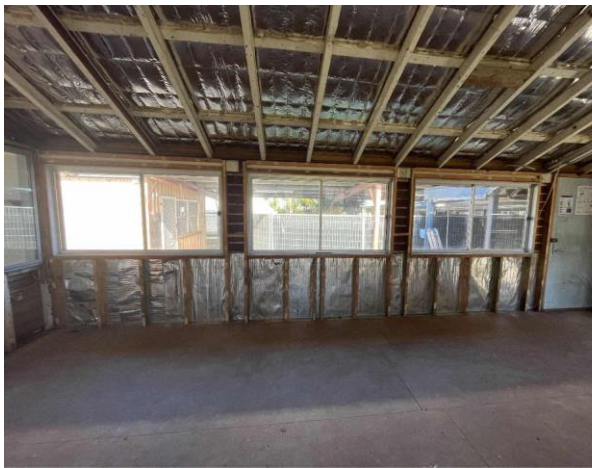
Line ID 62: Internal, Building A, Throughout, Walls, Sarking Insulation - Suspected SMF
