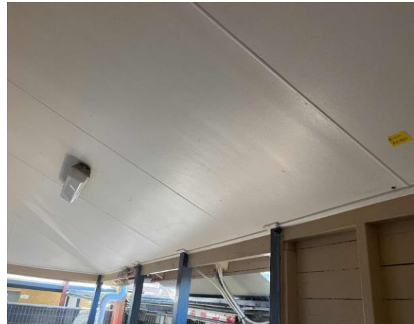
Line ID 4: External, Building E, Eastern Verandah, Ceiling, Fibre Cement Sheet - Chrysotile Asbestos Detected
