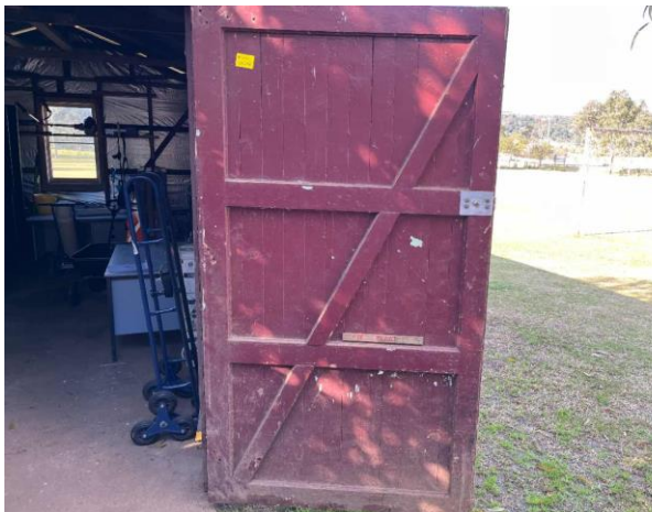
Line ID 49: Internal, Building D, Western Wall, Double Doors, Red (Dark) Paint - Lead Detected (0.054% w/w)
