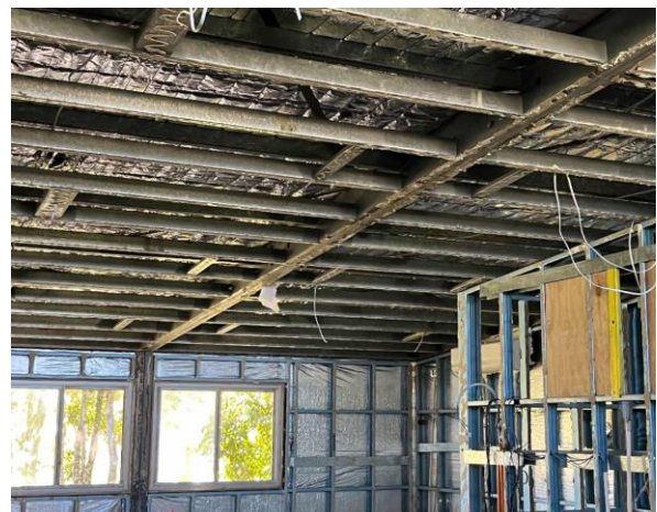
Line ID 65: Internal, Building I, Throughout, Debris to Ceiling, Insulation Batts - Suspected SMF
