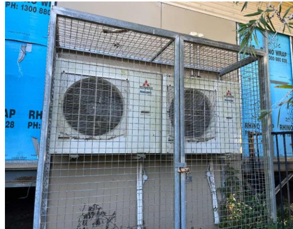
Line ID 73: External, Building I, Eastern and Western Sides, Mitsubishi Air Conditioning Units, R410A Hydrofluorocarbon (HFC) - Non ODS Refrigerant
