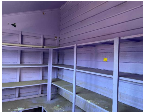
Line ID 51: Internal, Building E, South Eastern Storeroom, Walls and Ceiling, Purple Paint - Lead Detected (0.02% w/w)
