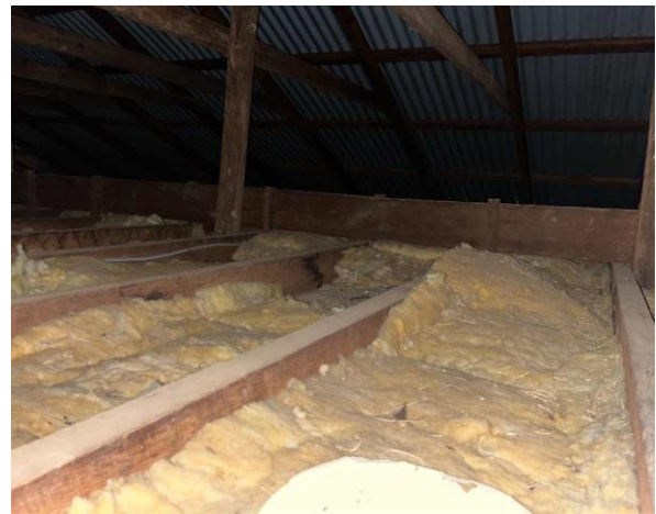
Line ID 63: Internal, Building E, Throughout, Ceiling Void, Insulation Batts - Suspected SMF
