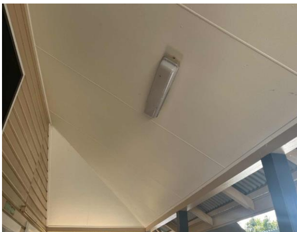
Line ID 70: External, Building F, East and West Verandah, Lights, Capacitor(s) - Non PCB Material
