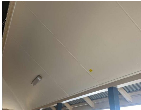
Line ID 8: External, Building F, East and West Verandah, Ceiling, Fibre Cement Sheet - Chrysotile Asbestos Detected
