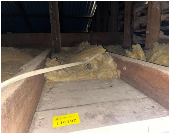
Line ID 60: Internal, Building E, Throughout, Ceiling Void, Dust - Lead Detected (2,600 mg/kg)
