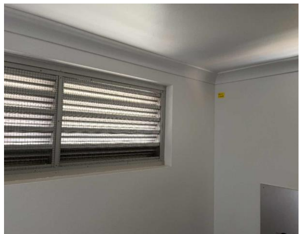
Line ID 59: Internal, Building J, Throughout, Walls and Ceiling, White Paint - Lead Detected (<0.005% w/w)
