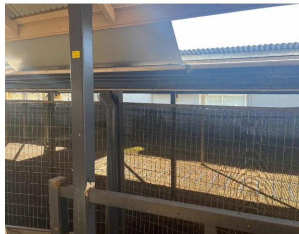
Line ID 40: External, Building F, Throughout, Handrails, Posts and Doors, Blue (Dark) Paint - Lead Detected (0.11% w/w)
