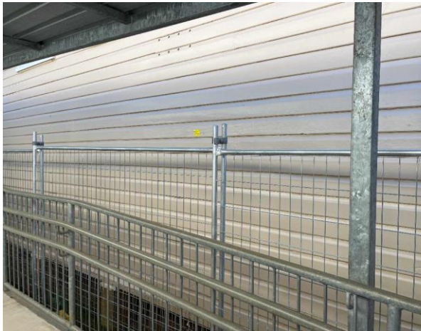
Line ID 41: External, Building F, Throughout, Walls, Beige Paint - Lead Detected (0.065% w/w)
