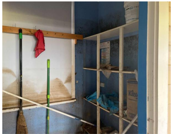
Line ID 57: Internal, Building F, Southwest Storeroom, Walls, Blue (Dark) Paint - Lead Detected (<0.005% w/w)
