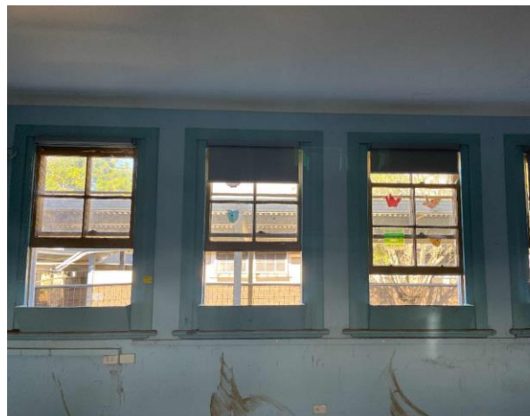
Line ID 53: Internal, Building E, Throughout, Window Frames, Blue Paint - Lead Detected (0.089% w/w)
