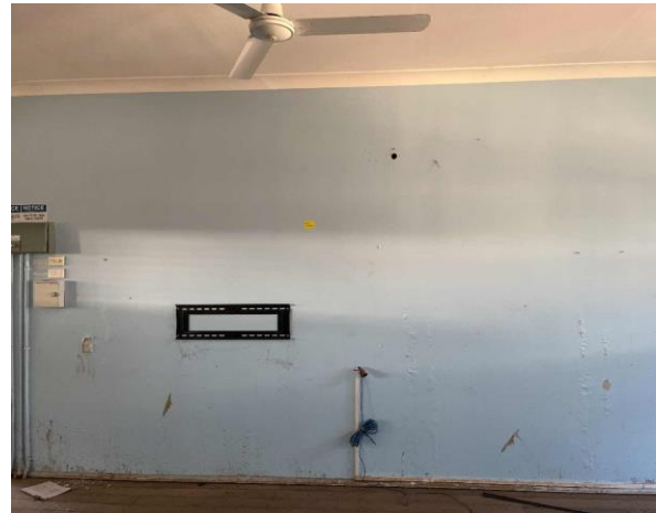
Line ID 23: Internal, Building E, Throughout, Walls, Fibre Cement Sheet - Chrysotile Asbestos Detected
