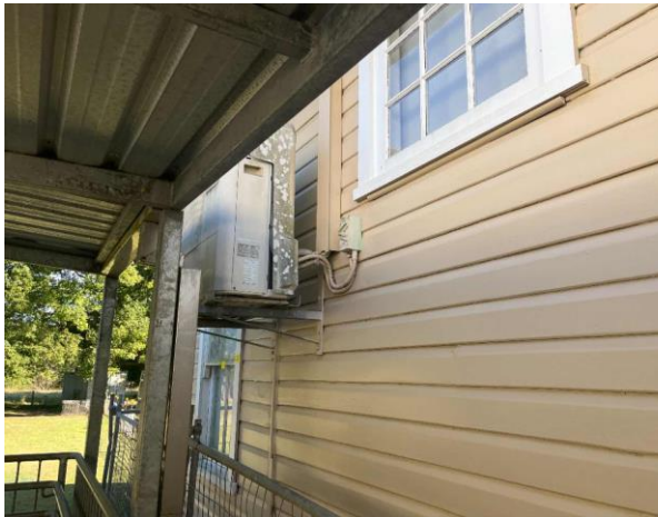
Line ID 72: External, Building F, South Side, Fujitsu Air Conditioning unit, R22 Hydrochlorofluorocarbon (HCFC) - ODS Refrigerant
