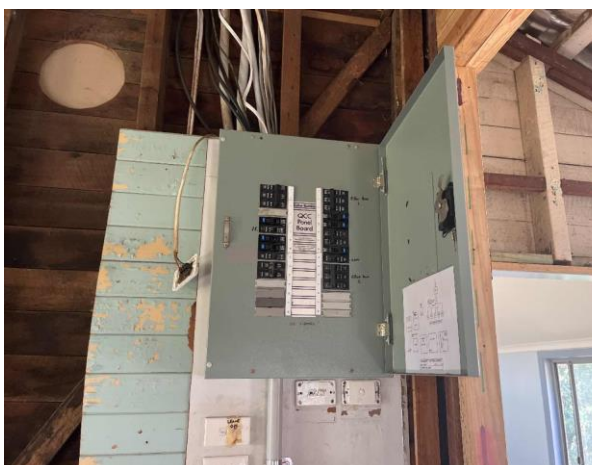
Line ID 18: Internal, Building A, Throughout, Switchboard, HRC Fuses - Suspected Asbestos
