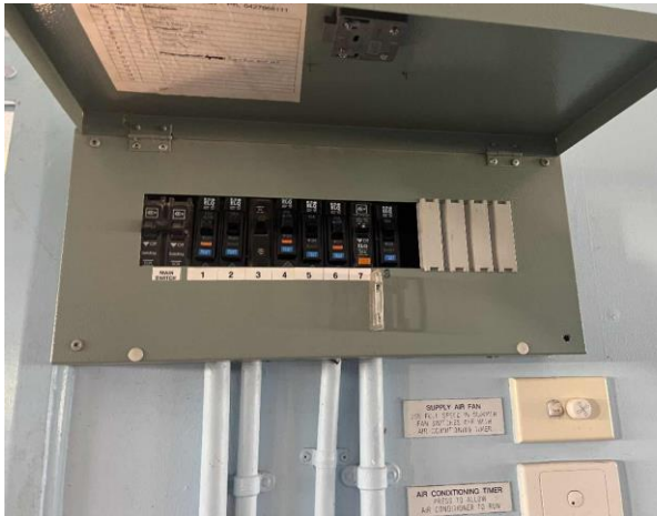
Line ID 22: Internal, Building E, Adjacent Entrance, Switchboard, HRC Fuses - Suspected Asbestos
