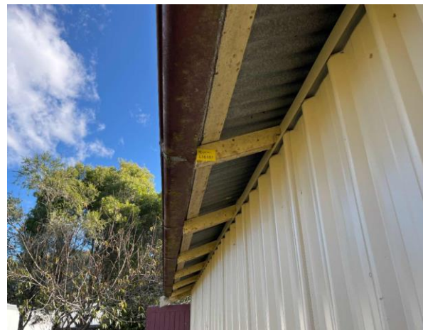
Line ID 34: External, Building D, Throughout, Window Frame and Wooden Frame Work, Beige Paint - Lead Detected (0.15% w/w)
