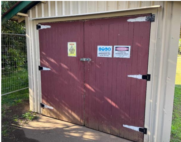
Line ID 35: External, Building D, Western Wall, Double Doors, Red (Dark) Paint - Lead Detected (0.054% w/w)
