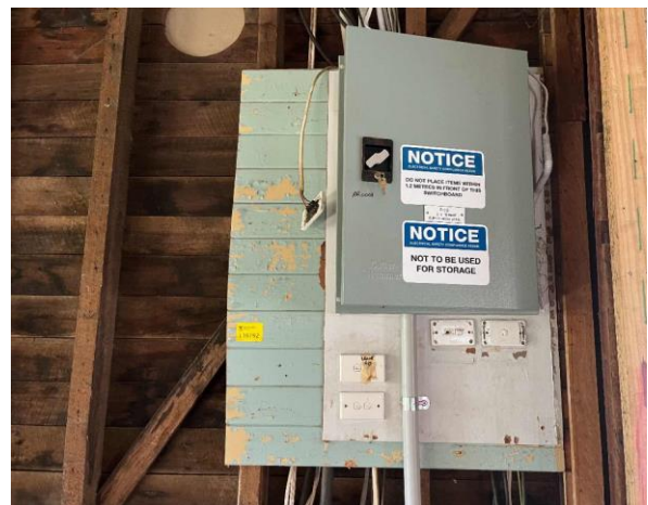
Line ID 46: Internal, Building A, Throughout, Panel Behind Switchboard, Light Blue Paint - Lead Detected (6.4% w/w)
